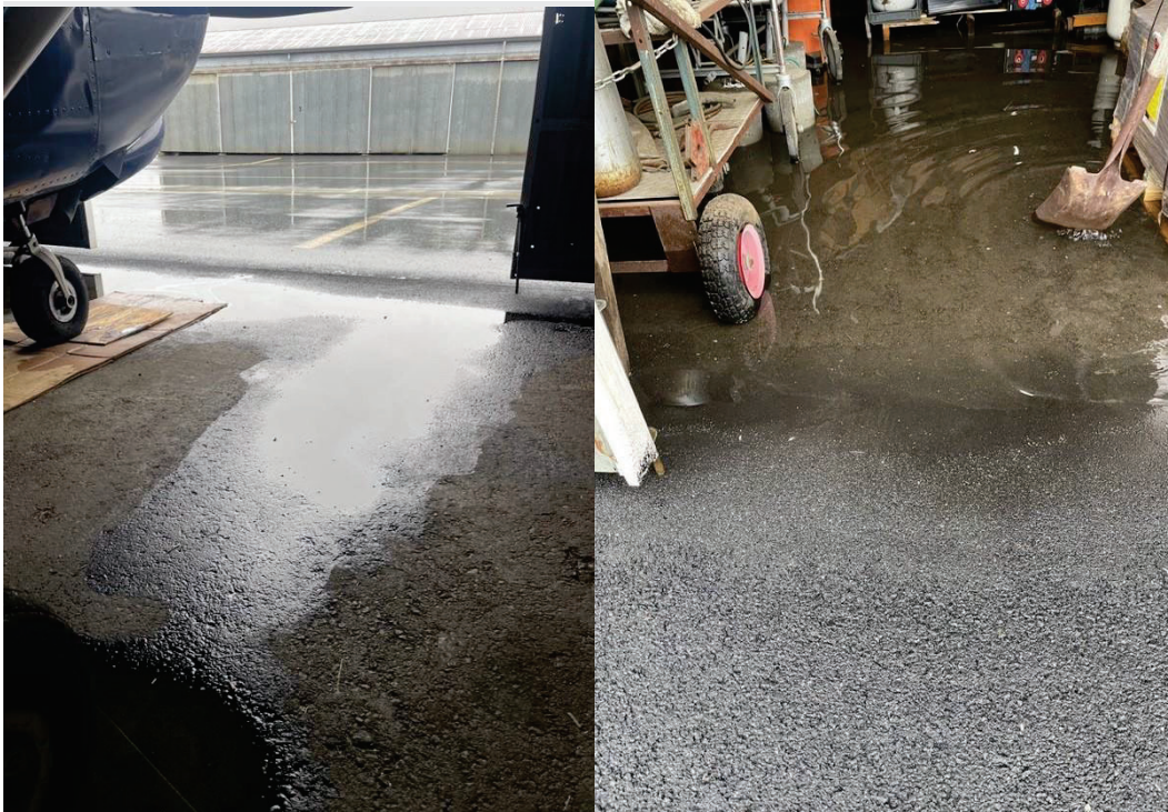
Pooling water problem in one of the Columbia Airport Hangars; Photo: Jury Member
