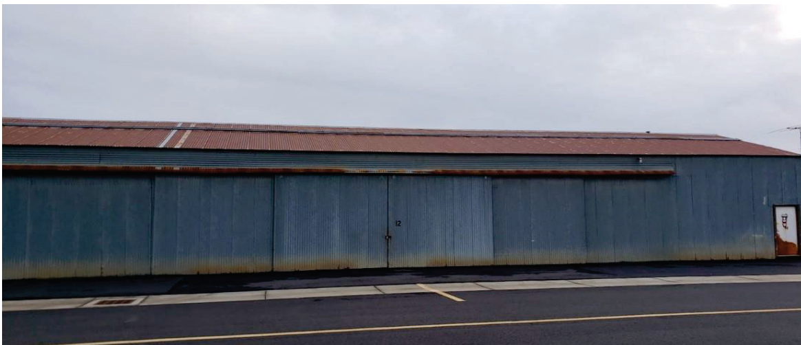
Rusted Roof, Sliding Door Hangars and Access Door; Photo: Jury Member
